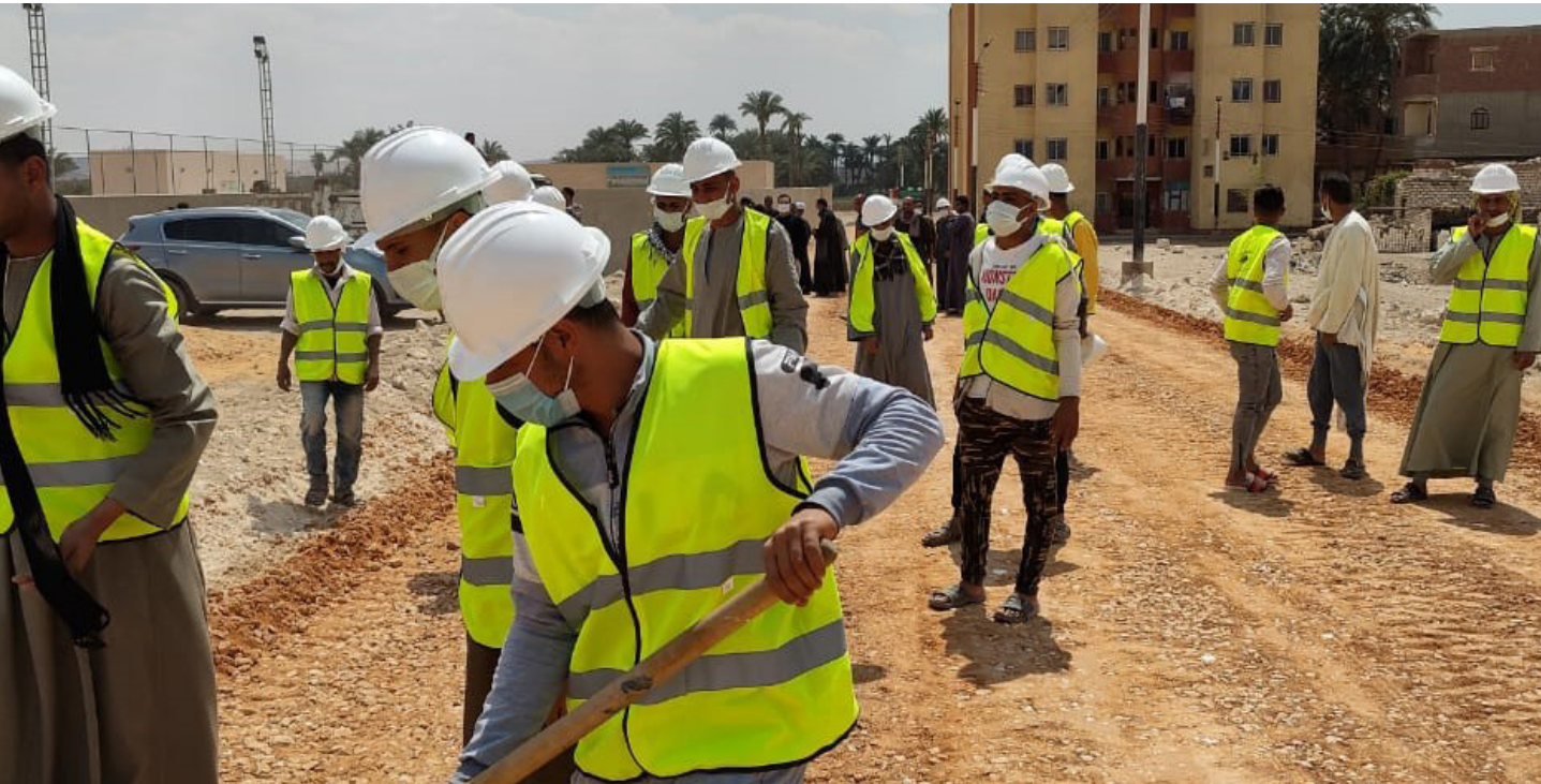
Rural road rehabilitation by MSMEDA in the Minya Governorate as part of the “Addressing root causes of irregular migration through employability and labour-intensive works” project, Photo: ©MSMEDA
