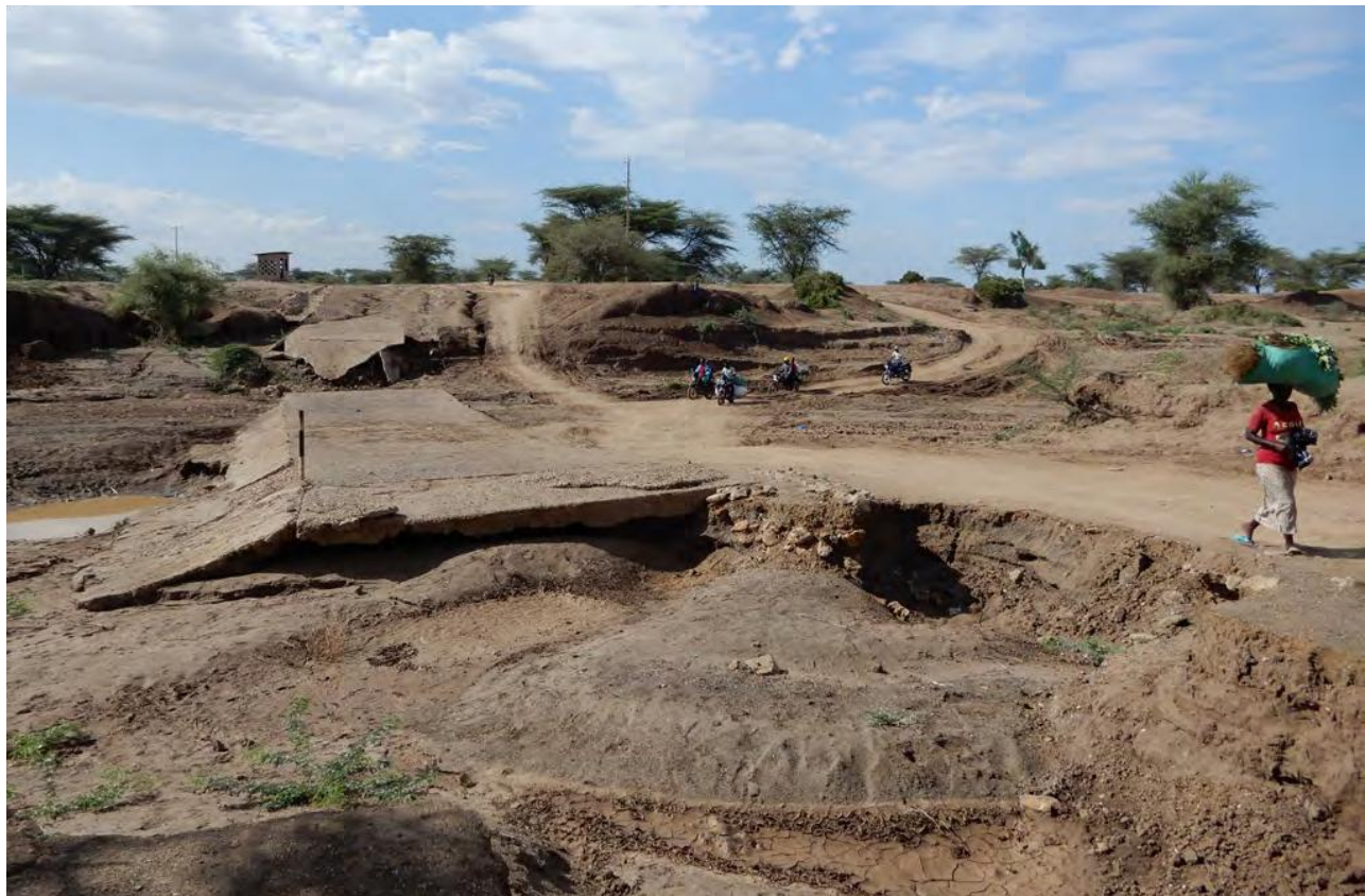
Fig. 33: Damaged Drift Near Fuji Primary School, Connecting Kakuma Camps 1 and 2 (UN-Habitat, 2023)
