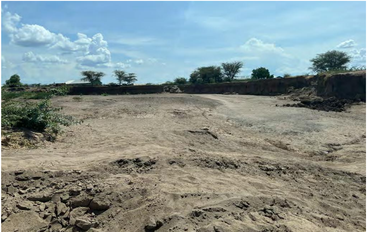
Fig. 40: Significant Erosion Along the Banks of the Lagga Between Kakuma Camps 1 and 2 (UN-Habitat, 2023)
